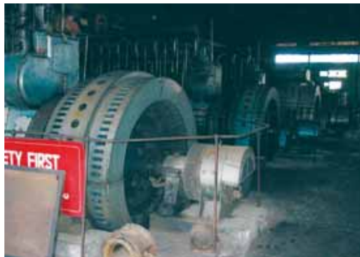
Site-tway's only source of electricity: colonial-era generators that provide just three hours of power a day
