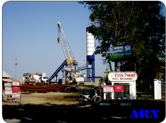
ESSAR company constructs Kaladan Multi Modal Transit Project in Sittwe, next to City Point restaurant
